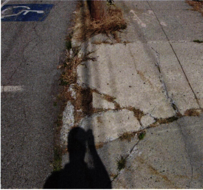
Front concrete pad needs removal & reconstruction.
