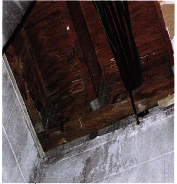
2 x 8 – 2 nd Floor roof joist – no insulation.
