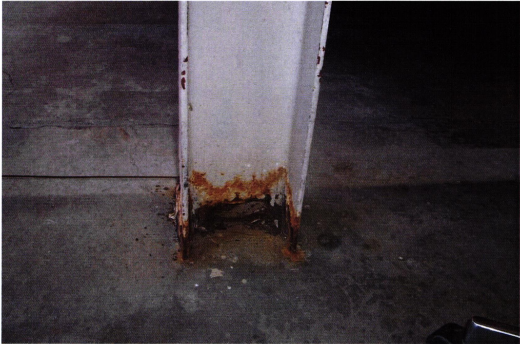
Photo 4.: Corrosion completely through the web of Apparatus Room steel wide-flange column.
