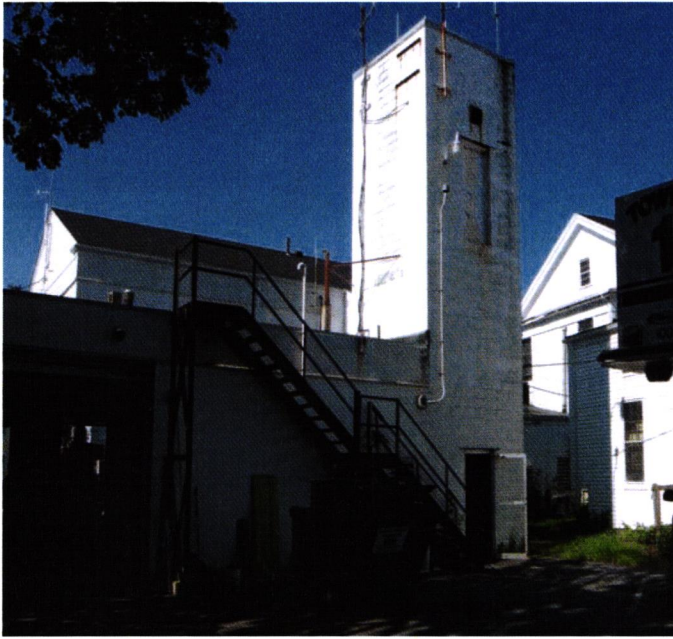
Stair not code compliant. Tower area.
