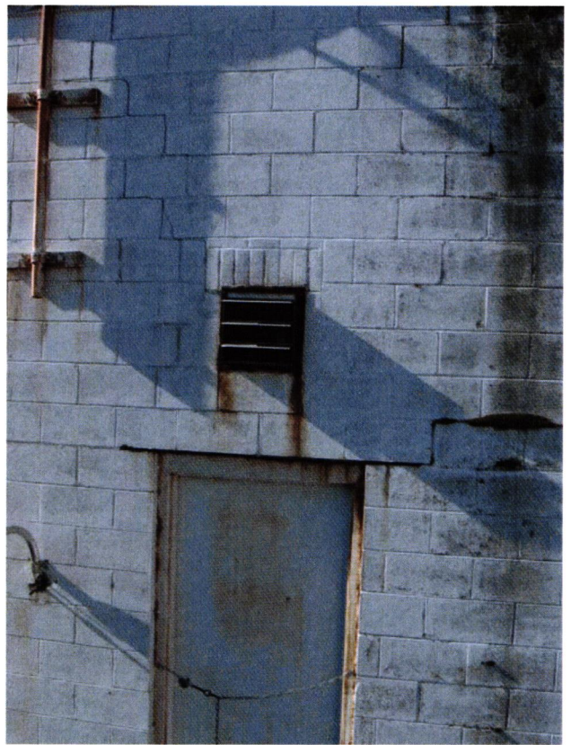
Water damage CMU.
