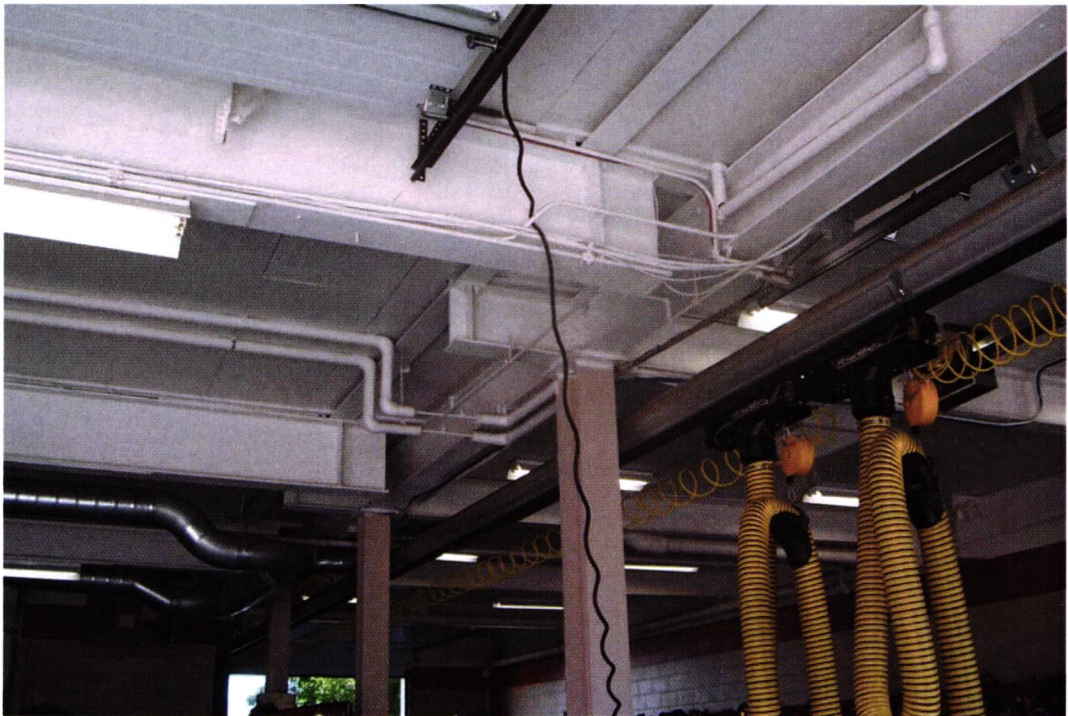
Photo 9.: View of ceiling of Apparatus Room, looking from front of station toward right rear corner. About midway between the black door track at the top center of the photo and the steel beam that extends from the upper right corner down to lower left, can be seen the bottom flange of a steel beam that is parallel to both. This steel beam is aligned with the east end wall of the Second Floor above. The rather complicated framing scheme seen in this photo was accomplished to allow the front-to-back columns line to be moved to the east a short distance, thereby allowing wider apparatus into this space.
