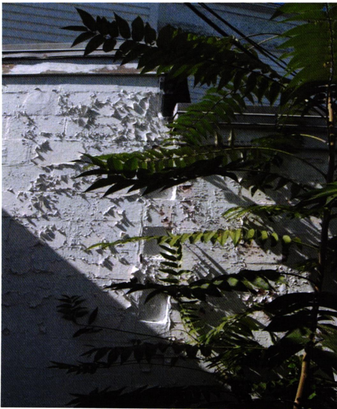
Paint peeling due to water entering block work.
