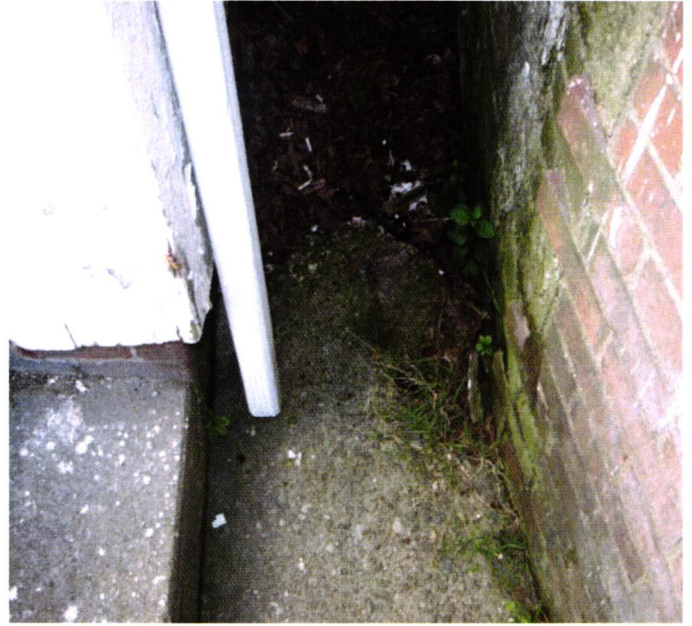
Water damage. Space between buildings.
