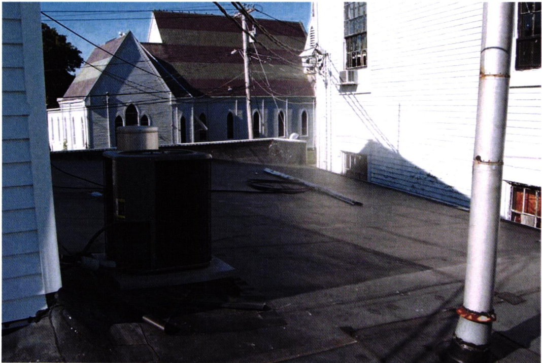
Photo 11.: View of low roof over one-story high west end of station, looking toward School Street. Note steeply-pitched roof for drainage.
