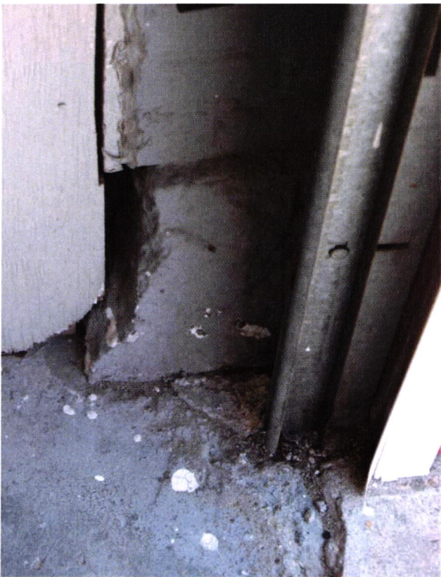
Block damage at overhead door.
