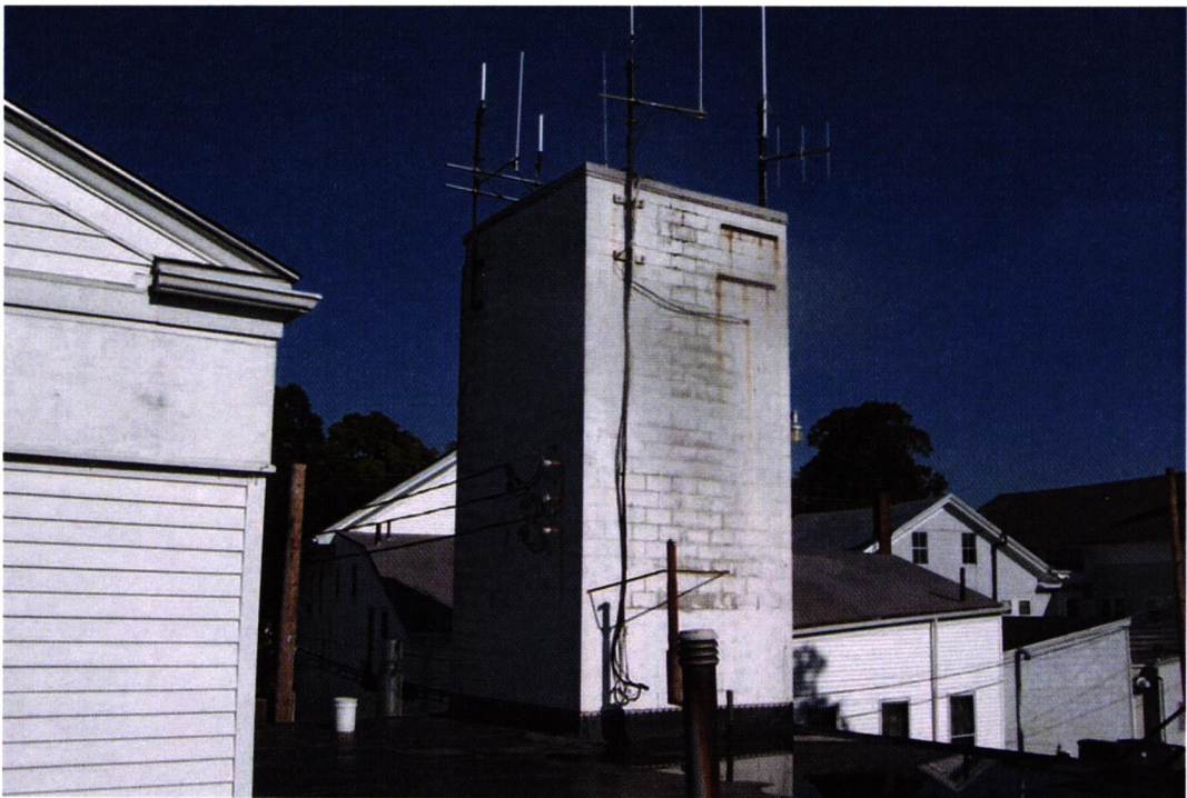
Photo 5.: Photo of Hose-Drying tower. Wood roof framing of the tower has deteriorated and suffered partial collapse, and masonry walls near the top of the tower show cracking and other damage.
