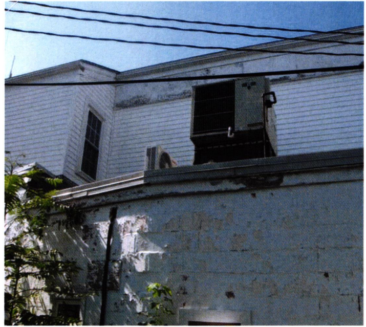
Water infiltrated CMU. Rotted trim.
