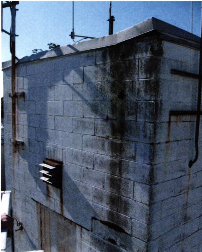
CMU block cracks and water leak.
