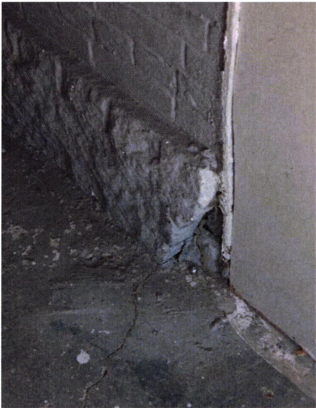
Cracked slab and granite foundation base.
