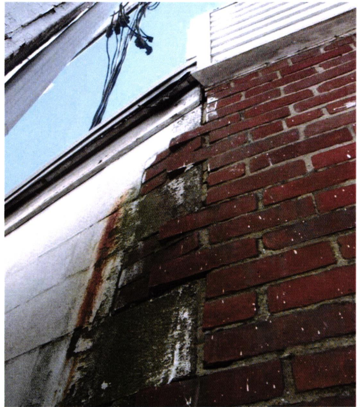
Mortar separation at brickwork and rotted trim.
