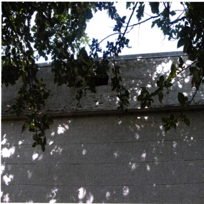
Wood band needs repair and repaint.
