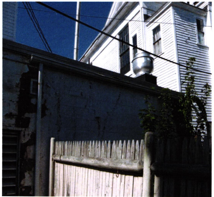
Roof flashing allowing water in block causing mortar to fail and paint to peel.
