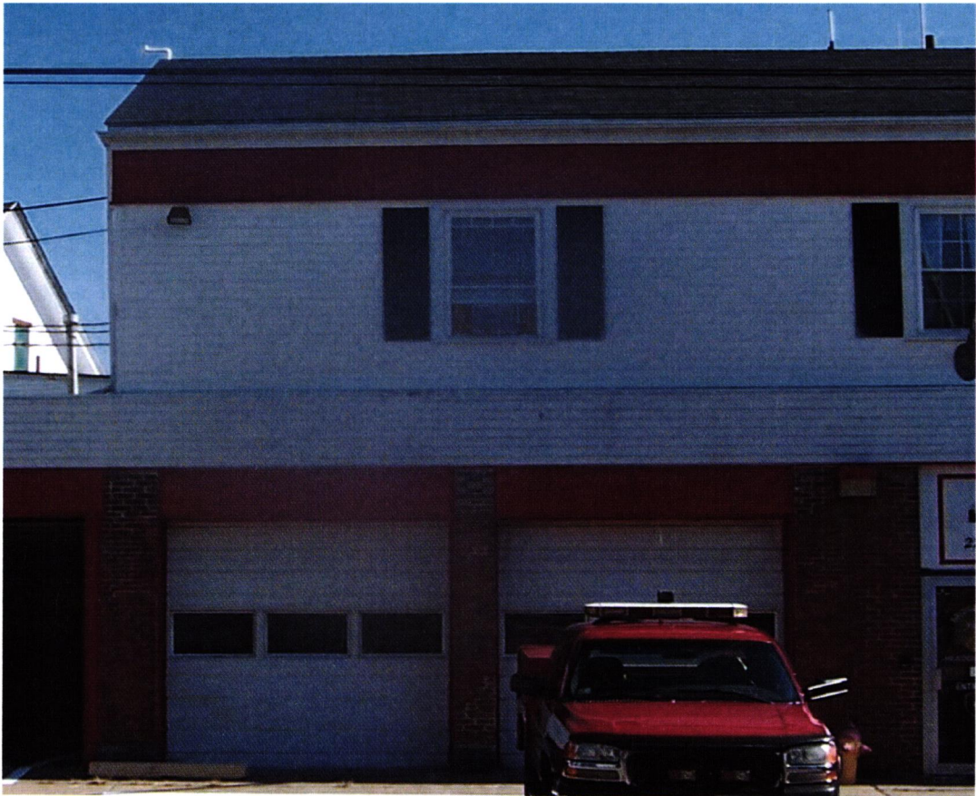
Photo 2.: View of the front section of the original two-story fire station, with the original vertical brick piers beside door openings still visible. What appear to be overhead doors are actually fixed-in-place panels, with interior finished office/command center space within. The Second Floor superstructure, above the low roof level (which is visible at left in the photo), is not original.
