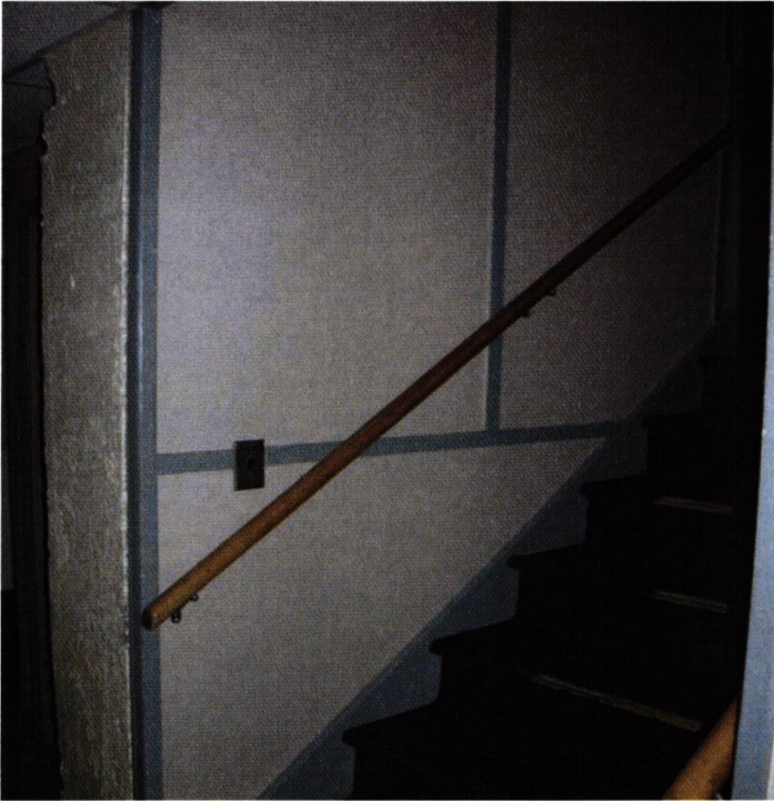
Wood stairs – not code compliant.
