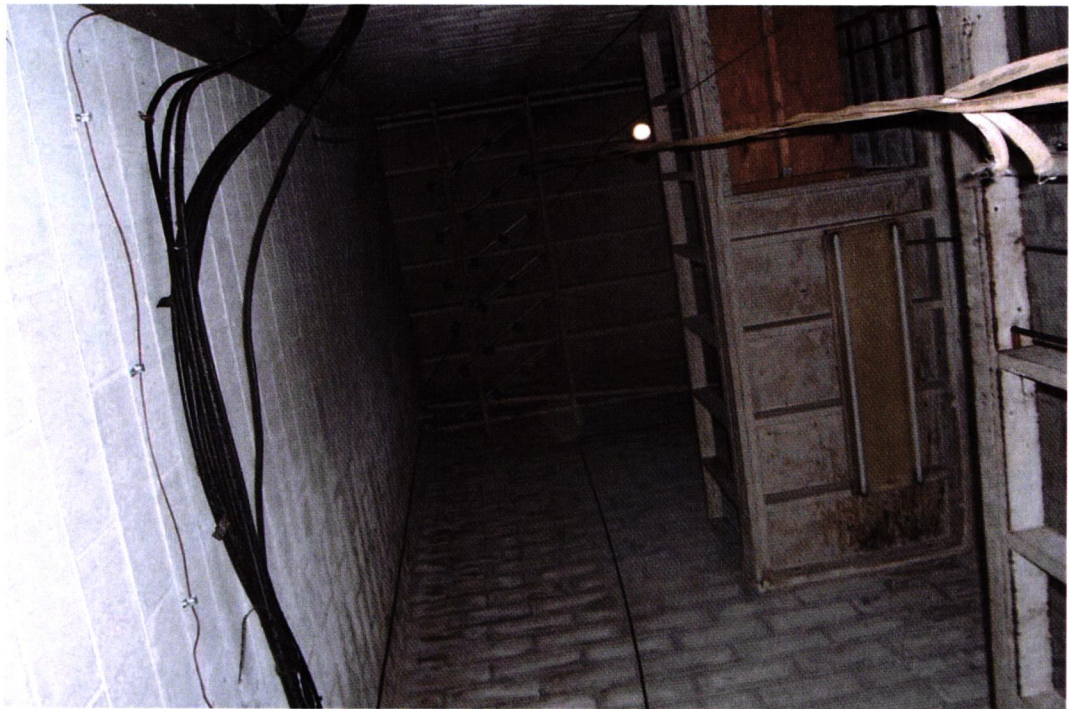
Photo 6.: View up into Hose-Drying tower from floor. Note second roof joist from bottom of photo is skewed, due to roof failure and partial collapse.
