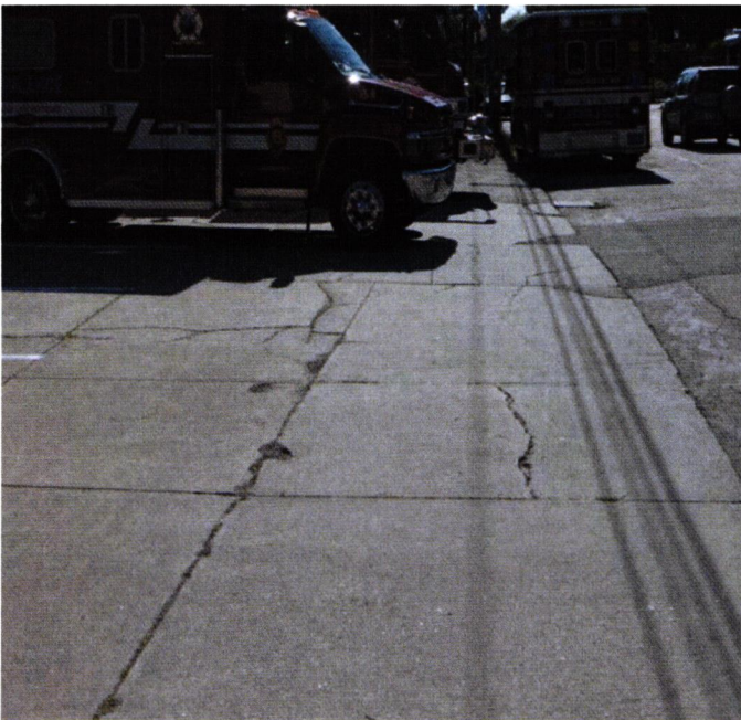
Cracks in concrete street pad.
