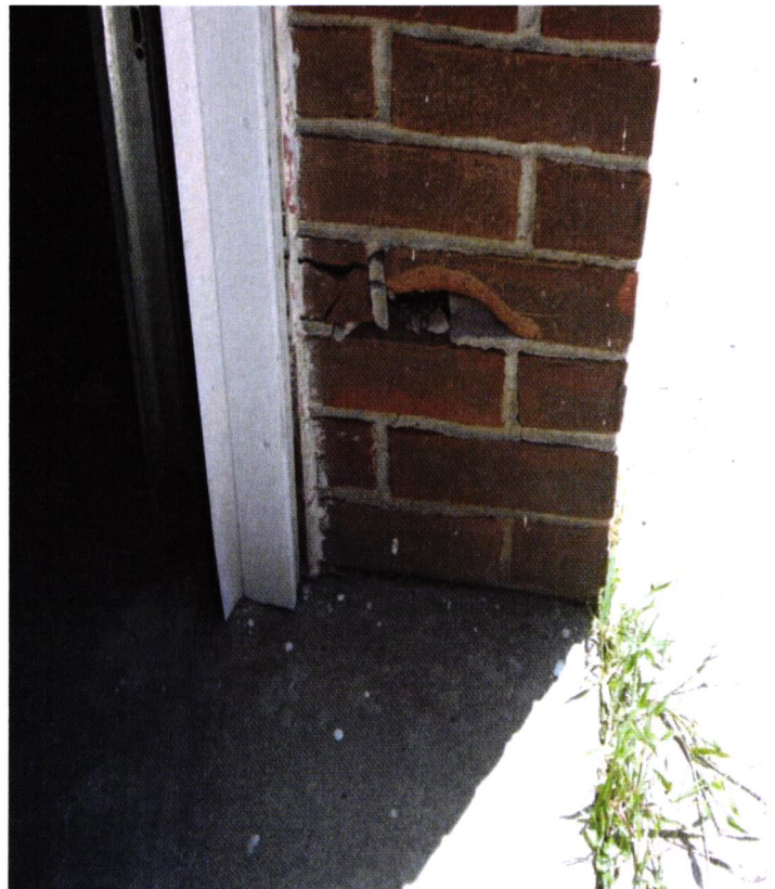
Brick damage at overhead door.
