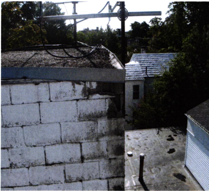
CMU damage at tower.
